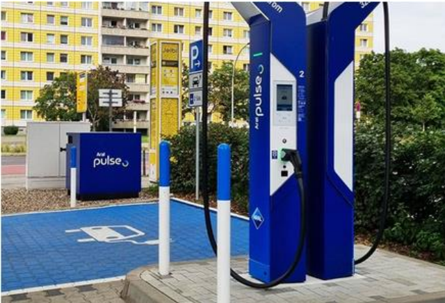
Exhibit 2: ChargeBox fast-charging point at Aral site in Germany
